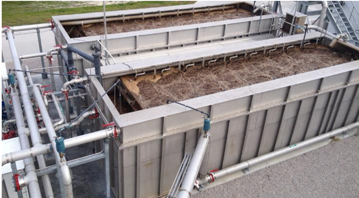
Figure 21: Image of a membrane bioreactor. It can be seen in this image that membrane bioreactors are similar in size to a shipping container (Evoqua, 2021).
