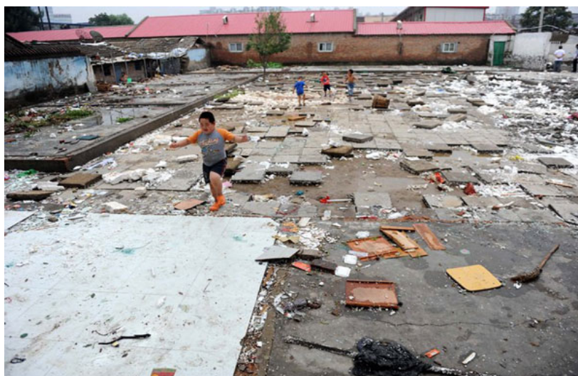
Picture 4. Migrant Children running through the trash after the demolition of migrant children school 14
